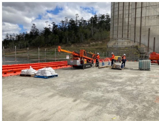
Figure 1: Works underway to set up the drill rig in preparation for passive anchor tests. The curved line of the original crest level can be seen on the wall of the left abutment in the distance.
